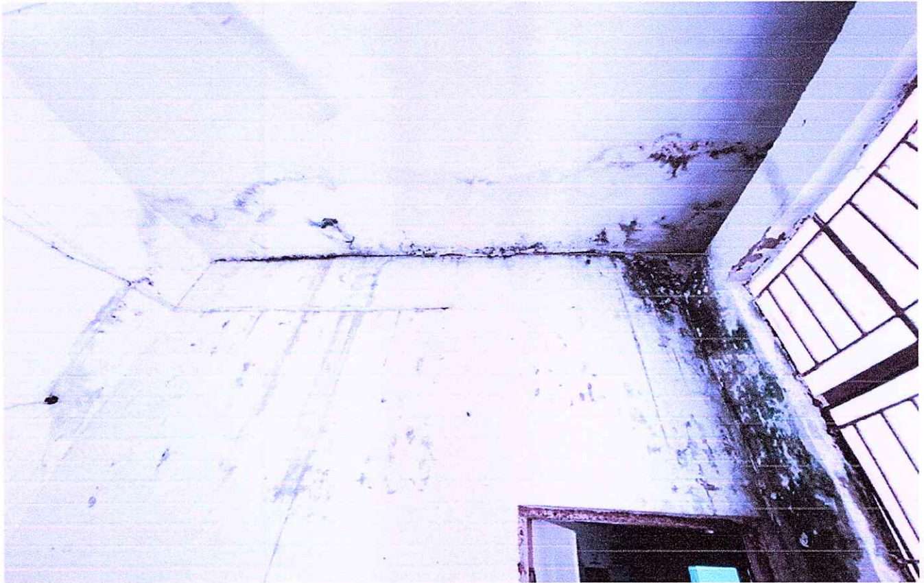
Major leakages has been observed on second floor at Chemistry lab where contact between slab and beam has been lost
