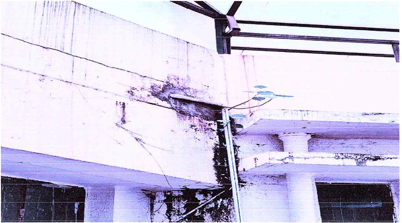
Vegetation Observed to parapet wall at open space in front of Library
